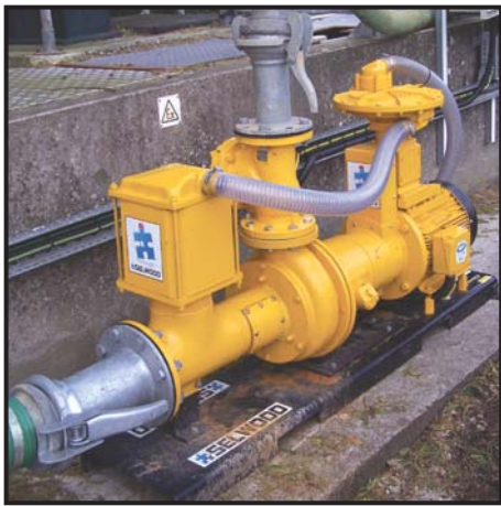
Sewage treatment works (UK) with SELPRIME
