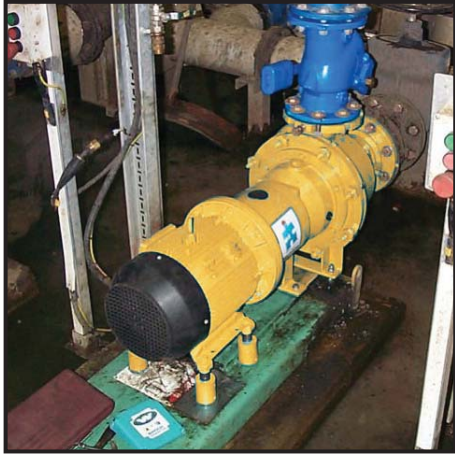
Sewage treatment works (UK)
