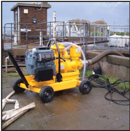
Sewage treatment works (UK)
